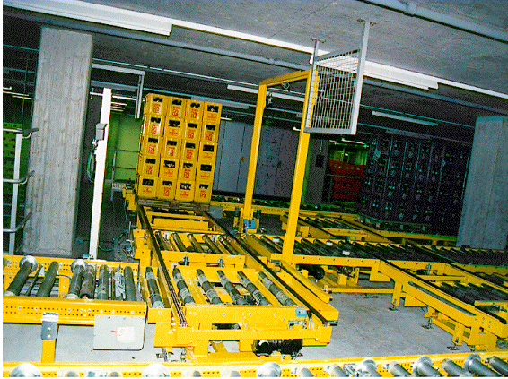
Figure 9: Conveyor System with I-Point
