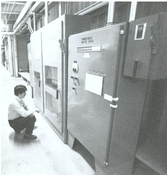
Design engineer Louis Cazenavette checks out a bank of A-B equipment. From the left are a Bul. 1373 DC drive and a Bul. 1790 unit which contains a 1774 PLC.
